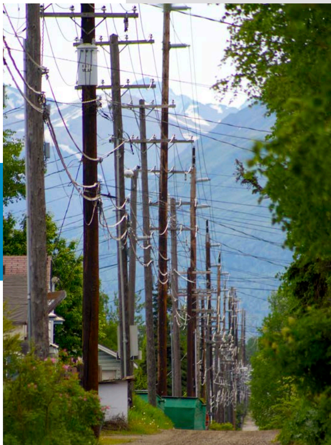
Power transmission lines near Anchorage, Alaska.
