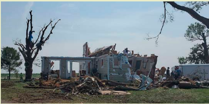
This house in Lake City, Iowa, was destroyed by an EF3 tornado on July 14, 2021.
